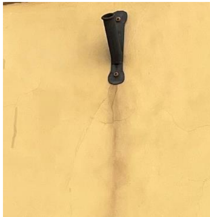
Figure 4.4 - Discoloration on the main façade
