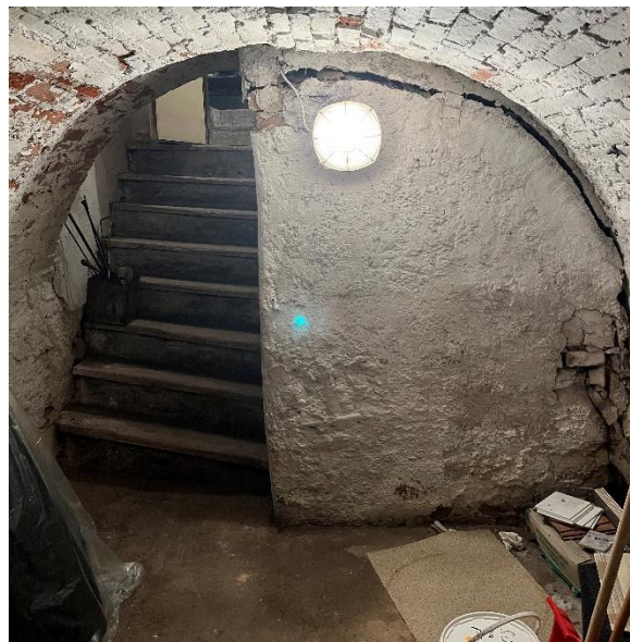
Figure 6.12 - The condition of the basement of the building
