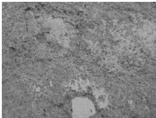
Fig. 8: Salt efflorescence at few mm from the outer surface pushing out plaster scales
