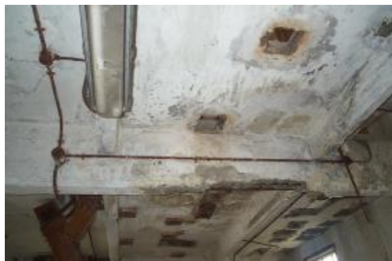
Fig. 2: Holes in the concrete floor, where the belts passed trough
