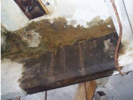
Fig. 4a: Damaged concrete
