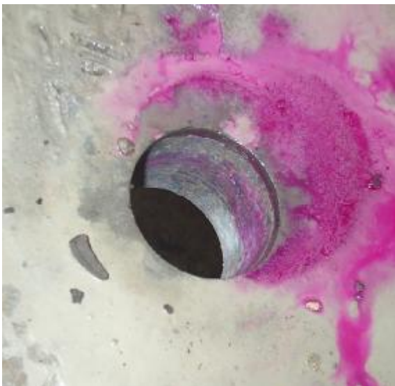
Fig. 5: Test results of phenolphthalein test on the hole of the drilled core number 23
